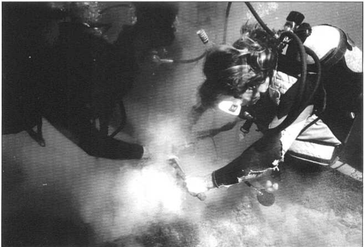
Figure 3-10. Reef mooring buoy installation involves the use of a hydraulic drill to remove a core from the fossilized coral bottom. A stainless steel eyebolt or u-bolt is inserted into the hollow core that is then filled with hydraulic cement to secure it to the ocean bottom. Next, a down line, round buoy float and pick-up line assembly are attached to the eyebolt. Pictured are divers drilling out the cores on the ocean bottom. Reef mooring buoys eliminate anchor damage to coral reefs. Buoys were first installed at Key West-area reefs by Reef Relief. (Photo: Craig Quirolo)
